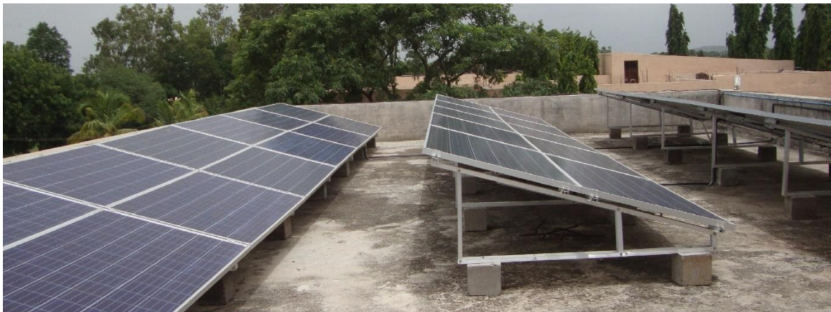
Roof top solar system
