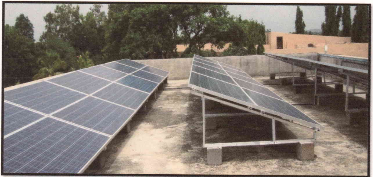
Roof top solar system
