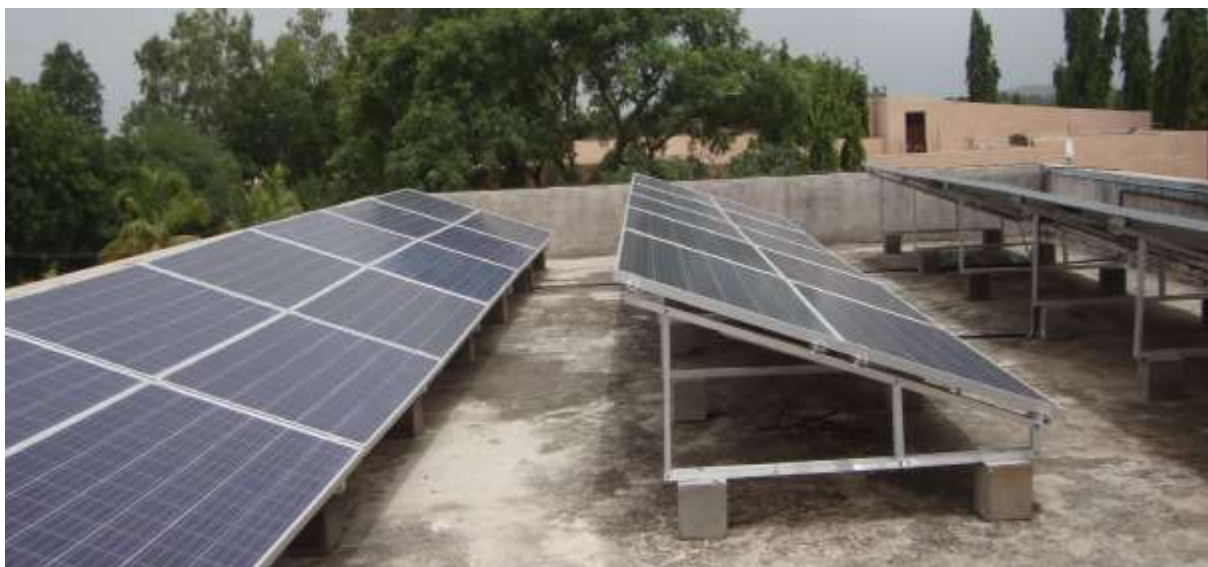
Roof top solar system
